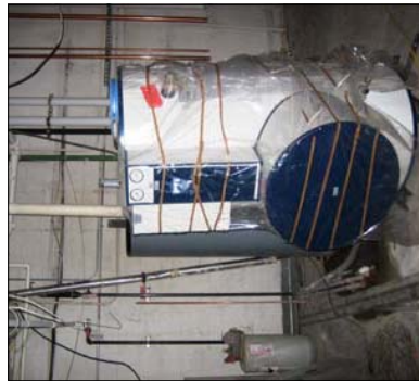
Mechanical Room Water Heater
