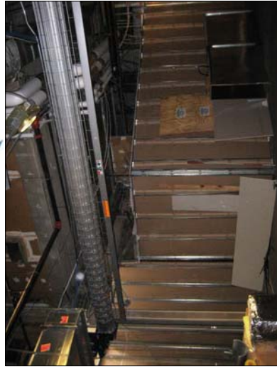
Coil Door in TSA Corridor
