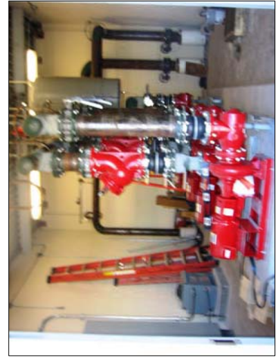
Painted Pump House and Equipment
