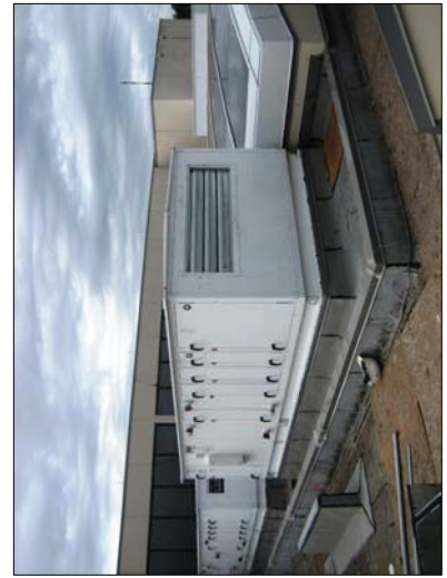
Roof top Equipment
